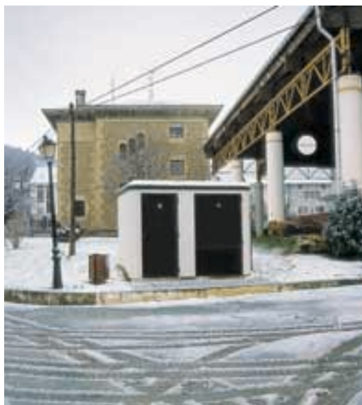
PFU-3 with 1 transformer
