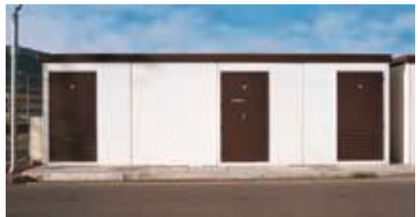
PF-204 with 2 transformers
