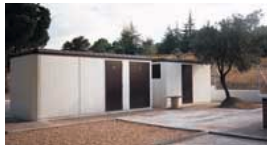
PFU-5 with 1 transformer and PFU-4 substation
