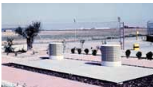
PFS-V exterior view of 1 Transformer.
