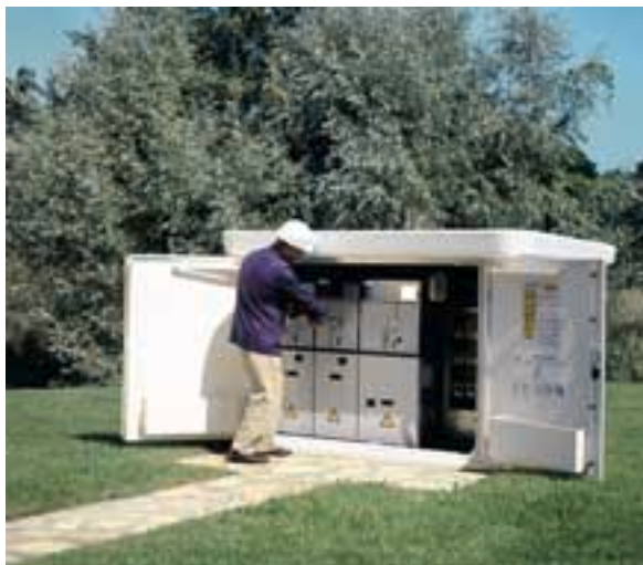
MV and LV switchgear in a MINIBLOK
