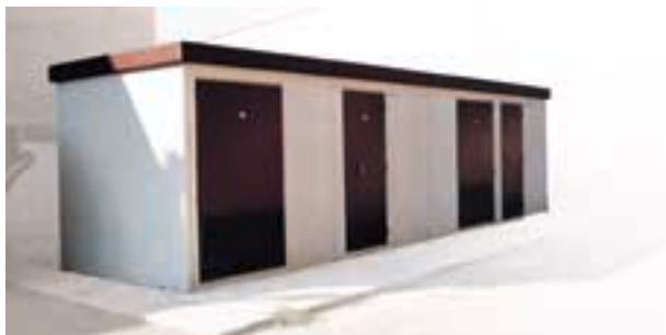
PF-203 with 2 transformers and PF-201 for metering
