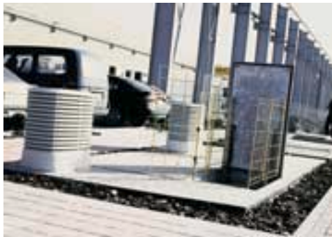
View of a PFS-V substation with the personnel access cover opened
