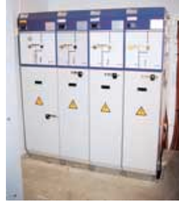
CGM 36 kV panels inside a PFS
